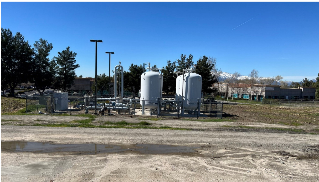
Facing west, nearby usage involving water distribution or irrigation, pumps.
